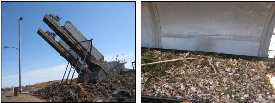
Figure 15. Biomass Fuel Being Unloaded at a Power Plant, Being Conveyed to Boiler
